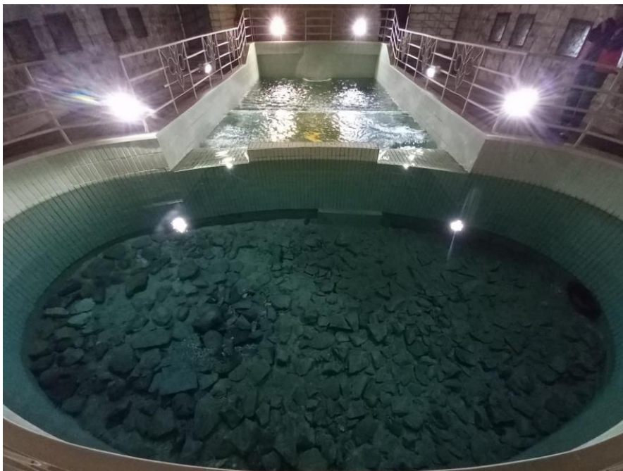
The inner part of the waterworks catchment facility of the Čierno II karst spring. Photo: Iveta Zvarová
