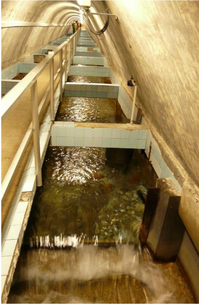
The flow measurement device (Poncelet's weir) at the end of the Lazce spring collection gallery. Photo: Peter Bajtoš.
