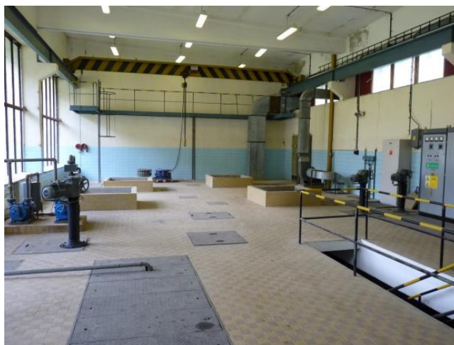
The interior of the Jergaly spring waterworks intake facility (Photo: Anton Auxt)
