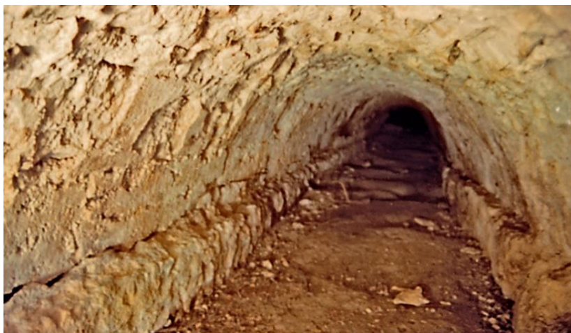
Remnants of the Hadrianic aqueduct. A bridge (top) and an underground conduit (bottom) of the aqueduct's structure in Nemea (after Lolos, 2010)
