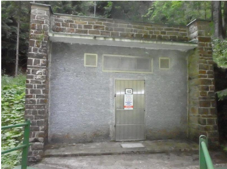
Entrance portal of the waterworks facility of the Bobrovecká dolina spring, managed by the Orava Water Company. Photo: Peter Malík.
