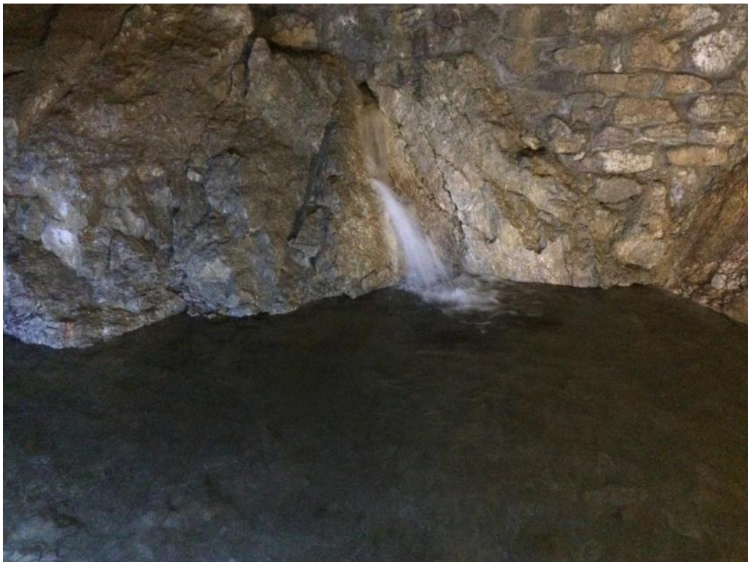
Groundwater discharging from fissures of scratched carbonates in the waterworks facility of the Bobrovec (Bobrovecká dolina) spring. Photo: Alexandra Vasilenková.
