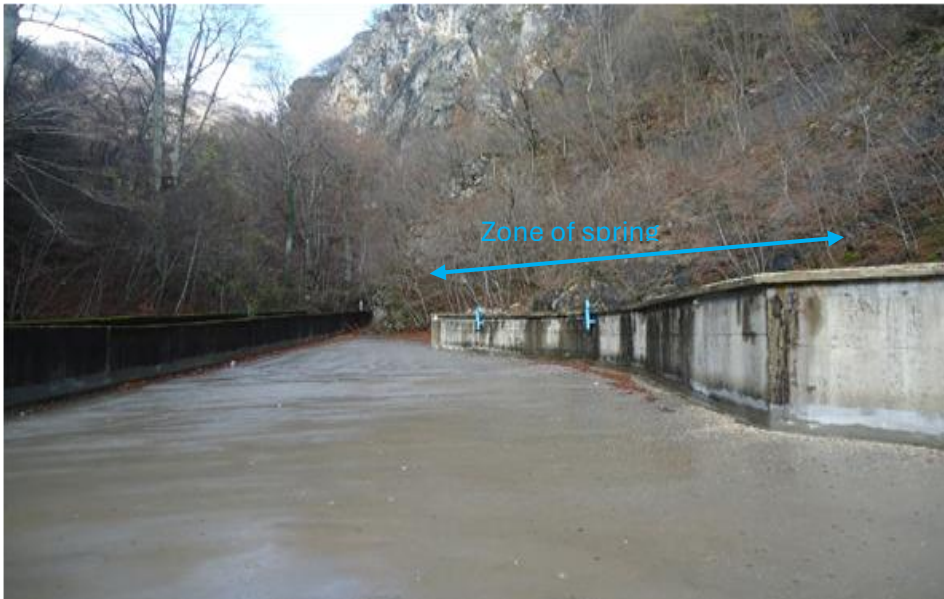
Reinforced concrete slab above the intake structure/collection channels and the spring of Studenchica
