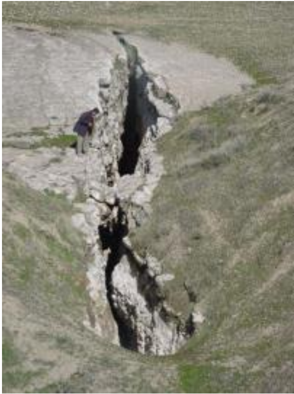
Deep crevasse / pothole expanded along long fault near Awa Spi (photo A. Iurkiewicz)
